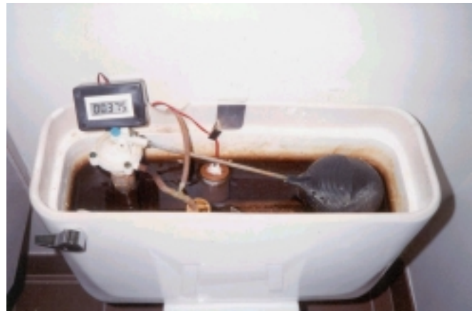
Figures 3 and 4 – Electronic flush counter connected to original toilet. Waterloo Landfill, Ontario
